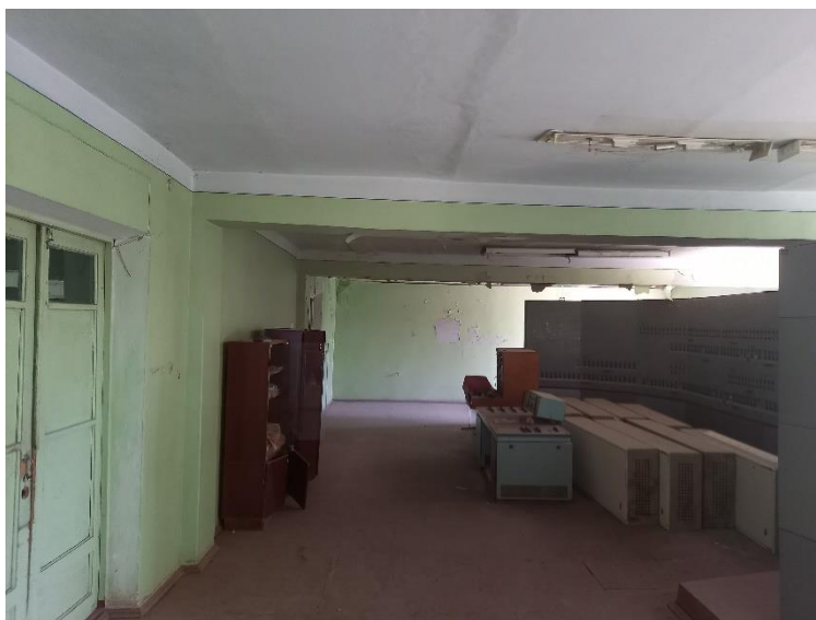
Photo. 17. Dysfunctional automated water distribution control desk on the TM-1 and TM-2 canals of the Zafarabad SRIA.
