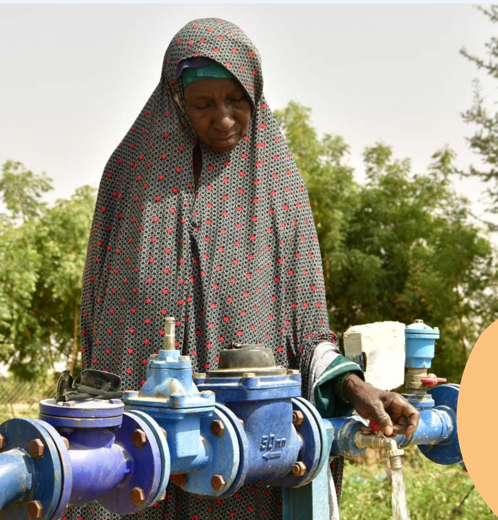
Image 6: The solar pumping irrigation system at the women's farming cooperative in Kollo © GIZ
