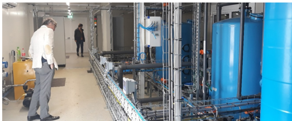
Black water treatment system
