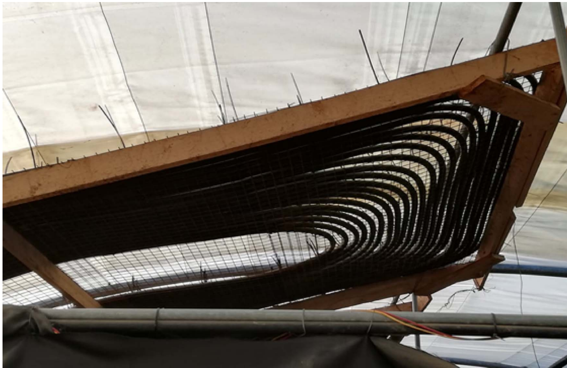
Figure 5. Solar thermal collectors in the 'Khodra'-Jordan facility.
