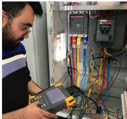
Figure 6: YWC Energy Team using energy audit mobile lab equipment (power analyzer)
