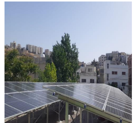
Figure 4: Wadi AlSeer 77 kWp PV system
